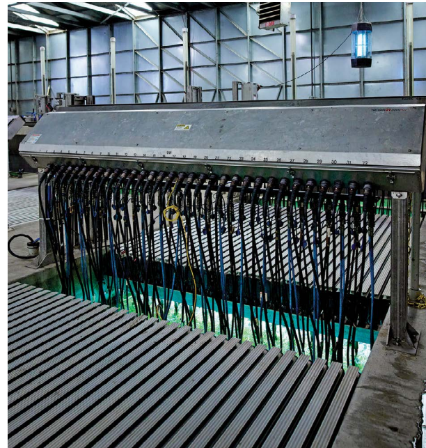
Treated water passes through a four-channel Trojan UV3000 Plus disinfection system before discharge to the Atlantic Ocean.
