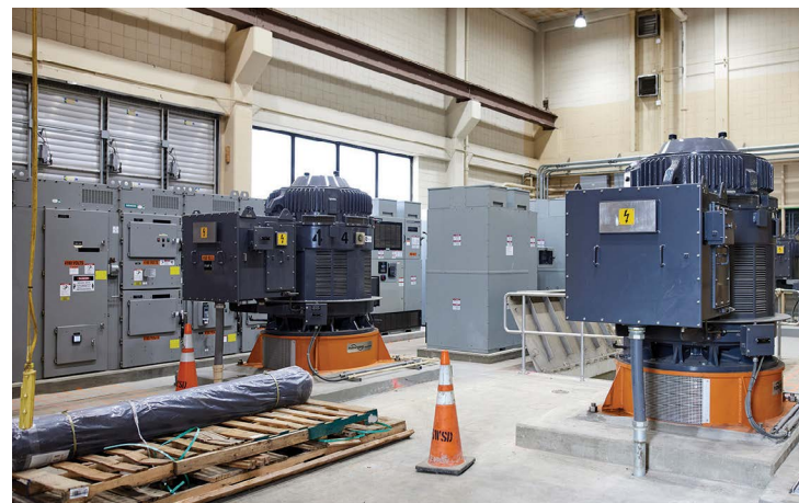
The pump room at the Bergen Point treatment plant includes pumps from Flowserve.
