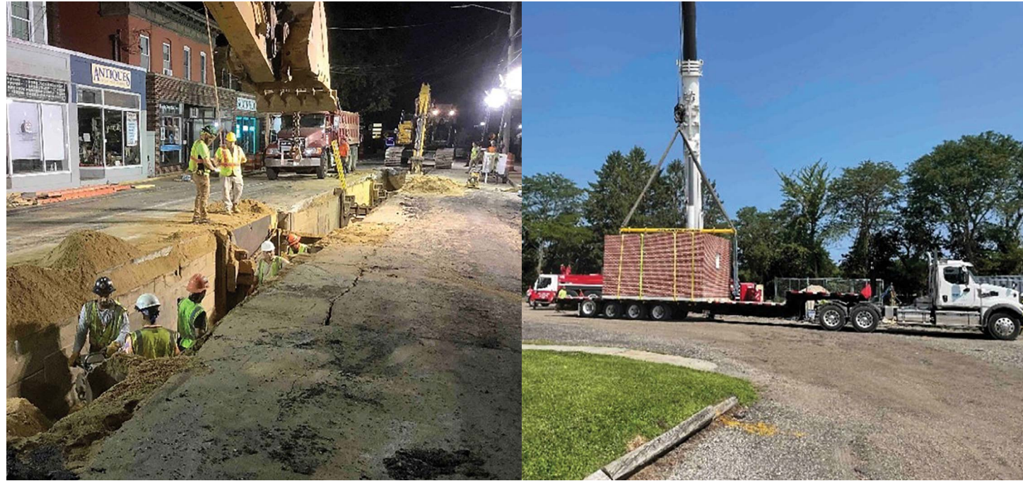
L-to-R Above: Sewer trench located in NYS 25A. Crane to set prefabricated pump station control building.
