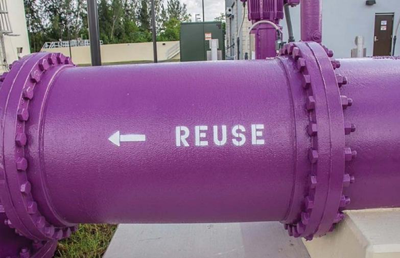
Purple pipes carrying reclaimed water in Florida. Credit: Sawgrass Wastewater Treatment Plant, City of Sunrise, Florida
