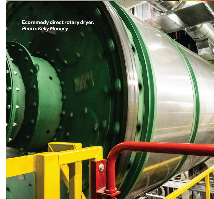
Allen Bradley control board. Photo: Kelly Mooney
