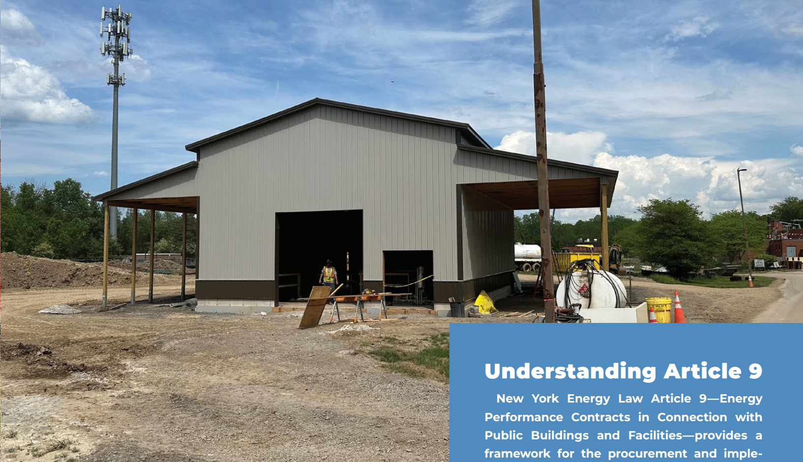
The new outside waste acceptance building will include a new Saveco Beast unit to screen debris from septage and grease interceptor waste. The two tanker discharge lanes will allow the plant to accept outside waste for either co-digestion or treatment through the liquid treatment stream, while keeping all of the truck traffic out of the main treatment area. Photo: Dennis Clough
