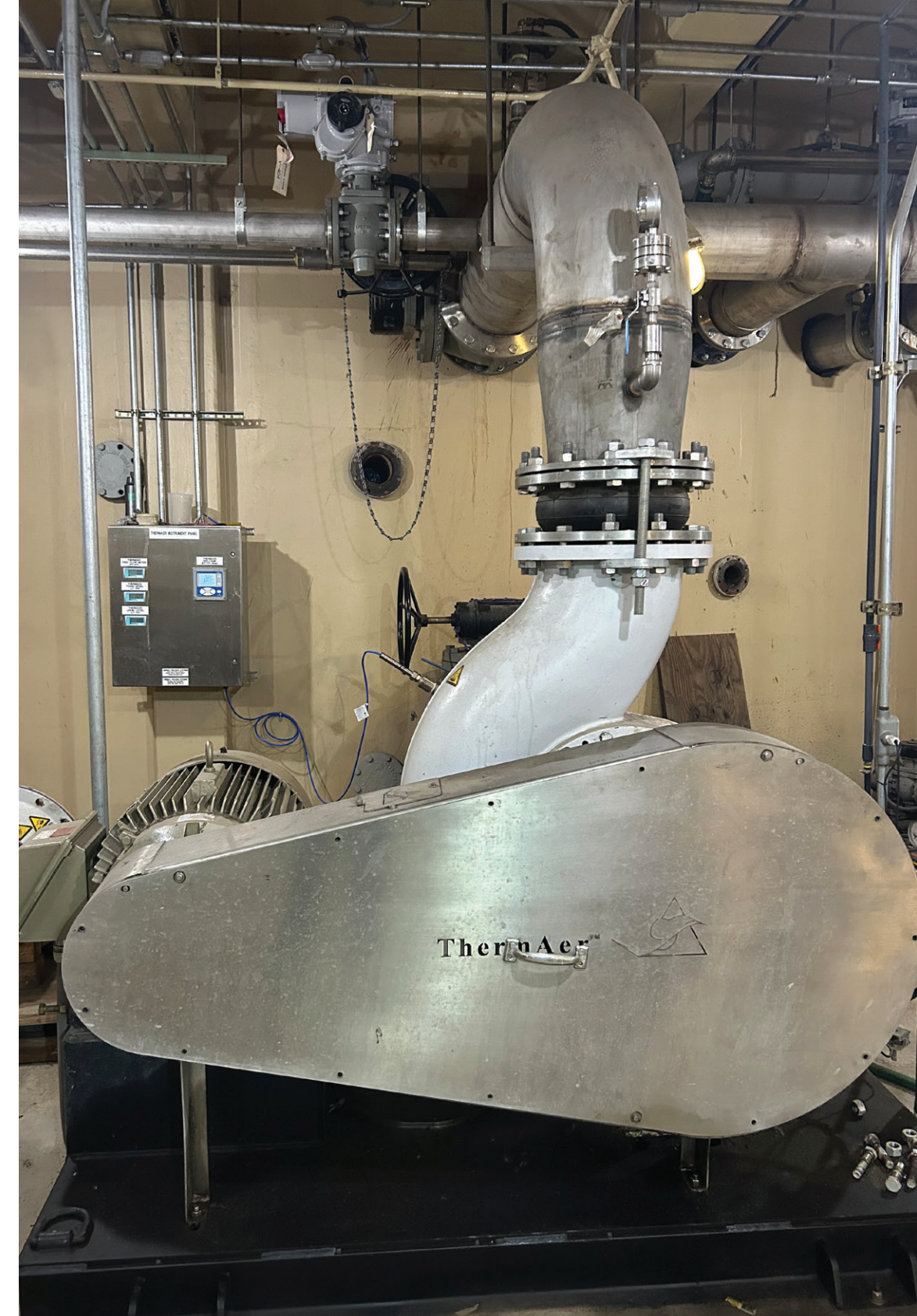
Photo 3. The Thermaer mixing pump typically runs constantly to keep the reactor thoroughly mixed, creating the largest electrical load of the ATAD system. Photo: Tim Carpenter
