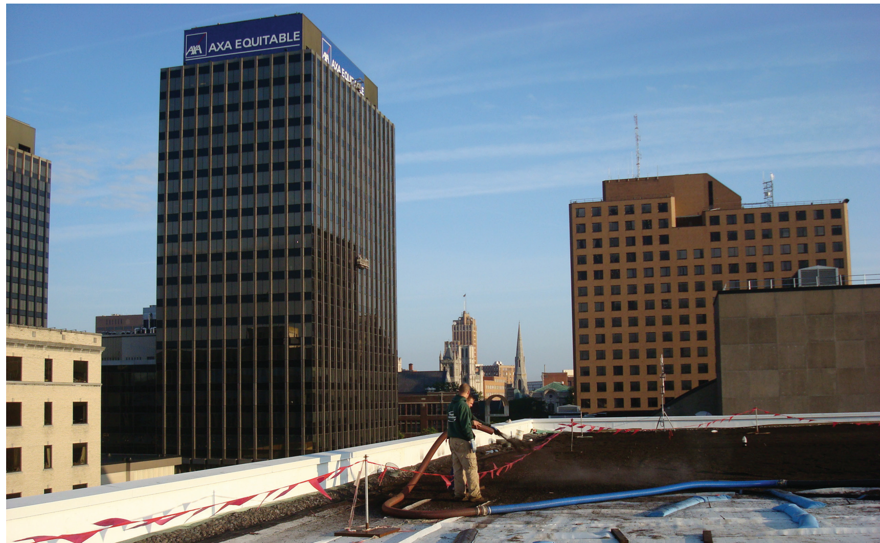
Green roof growing media is installed at the Oncenter in Syracuse, New York. Photo: Denali
