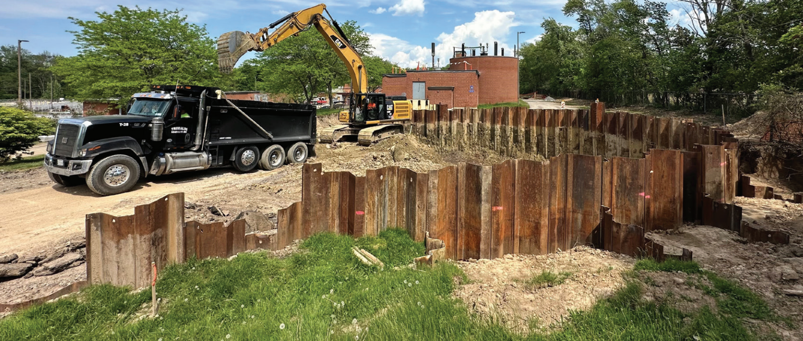
Excavation for the foundation of the new 1.15-million-gallon primary anaerobic digester. The site constraints and soil conditions required the use of sheeting to support the excavation. Photo: Dennis Clough
