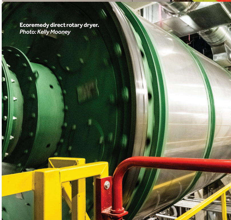
Allen Bradley control board. Photo: Kelly Mooney
