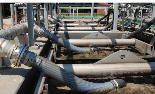
Aqua-Aerobic® MBR System at Riverhead, NY
