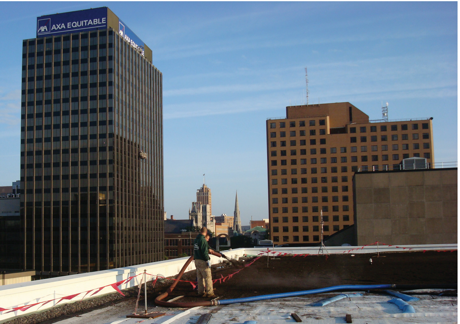
Green roof growing media is installed at the Oncenter in Syracuse, New York. Photo: Denali
