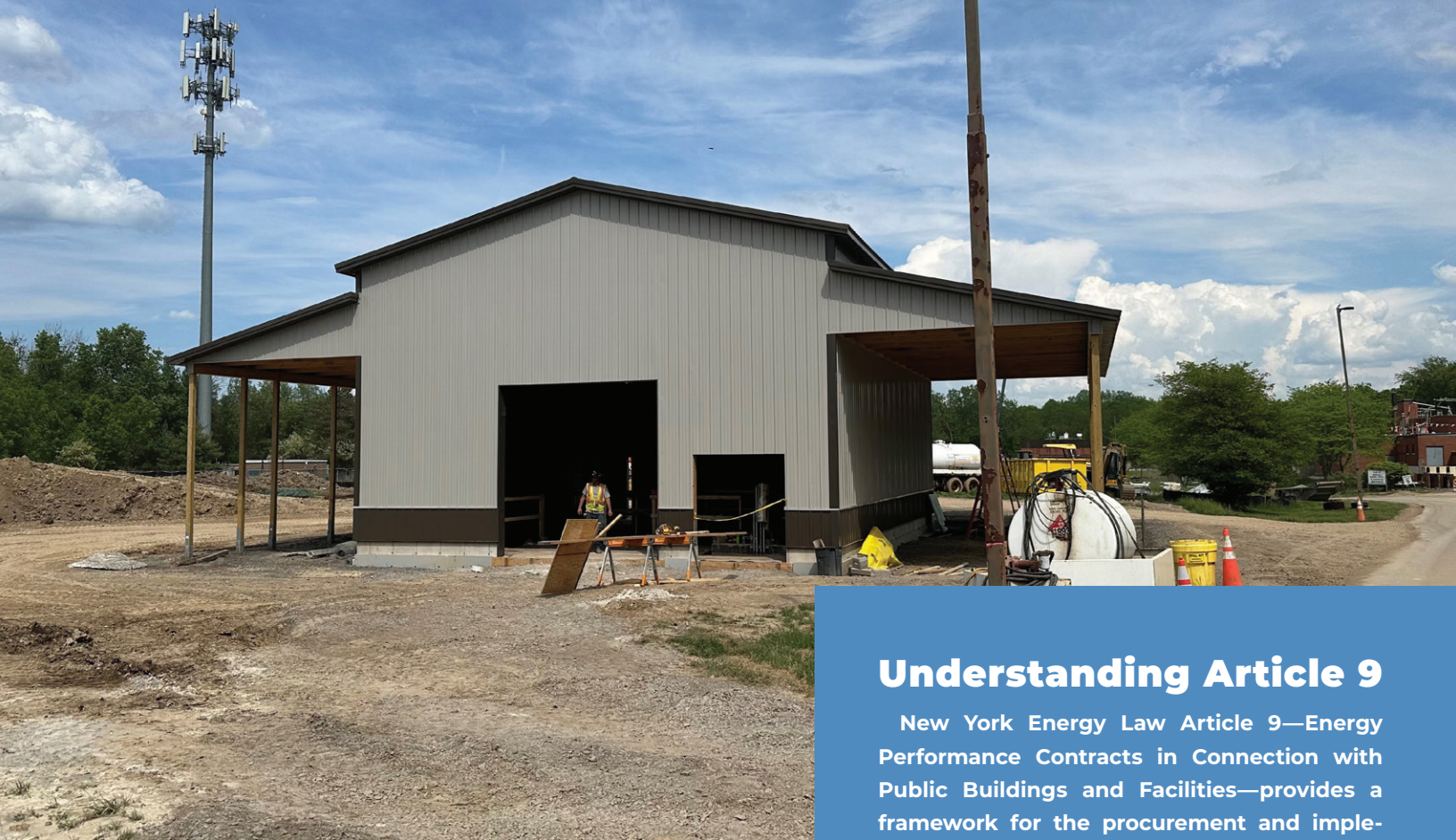
The new outside waste acceptance building will include a new Saveco Beast unit to screen debris from septage and grease interceptor waste. The two tanker discharge lanes will allow the plant to accept outside waste for either co-digestion or treatment through the liquid treatment stream, while keeping all of the truck traffic out of the main treatment area. Photo: Dennis Clough
