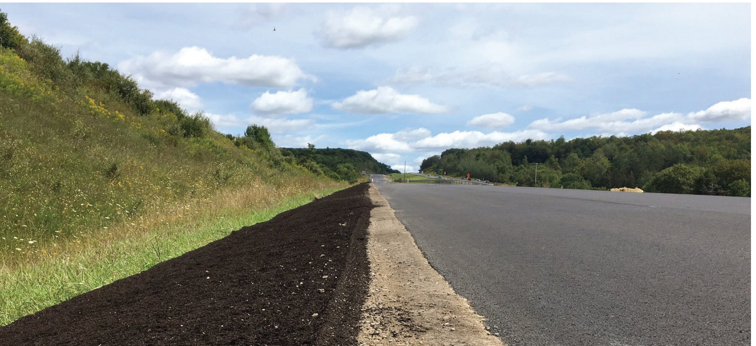
Biosolids compost being applied for miles along the side of a New York state highway project to promote the establishment of vegetation. Photo: Denali
