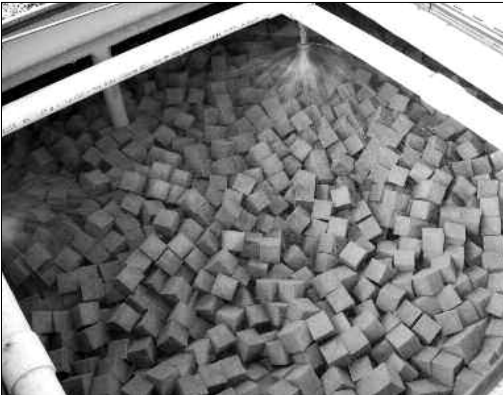
Attached growth bioreactor: foam blocks with settled wastewater sprayed over the top. Attached growth microbes live on the foam blocks, which provide increased surface area for more biomass to grow.
