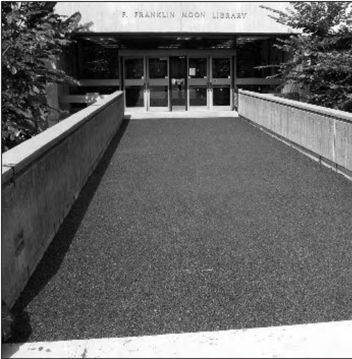
Porous pavement walkway made from recycled rubber leads to the Franklin Moon Library at SUNY-ESF.
