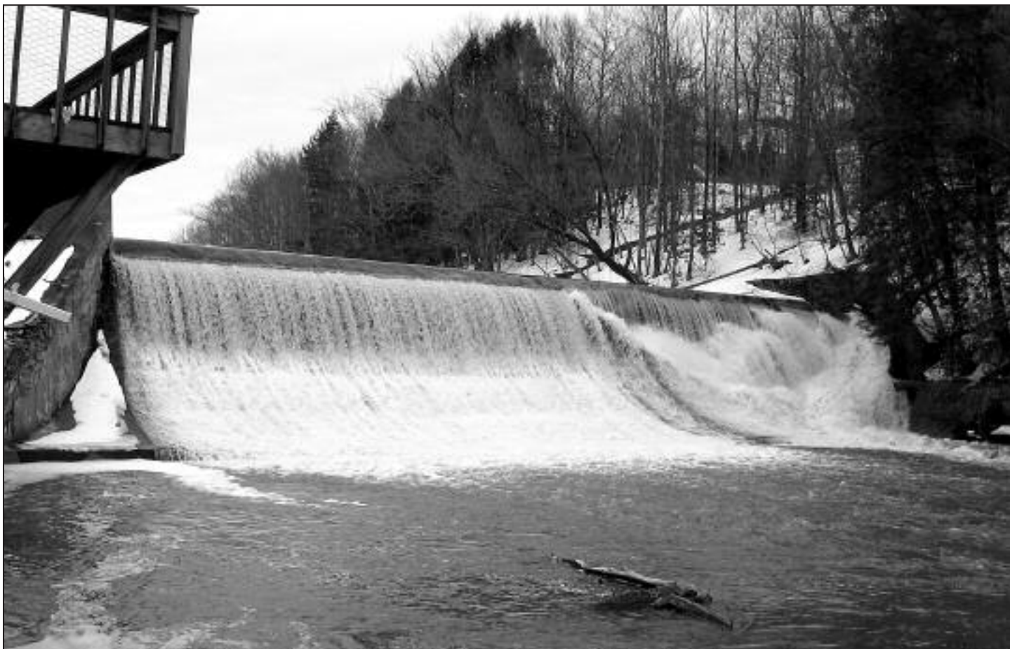
Concrete overflow spillways may become worn over time.
