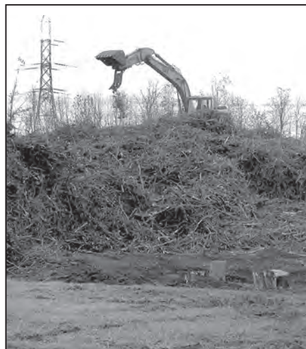
Tonawanda, NY compost site moving debris already put through the tub grinder
