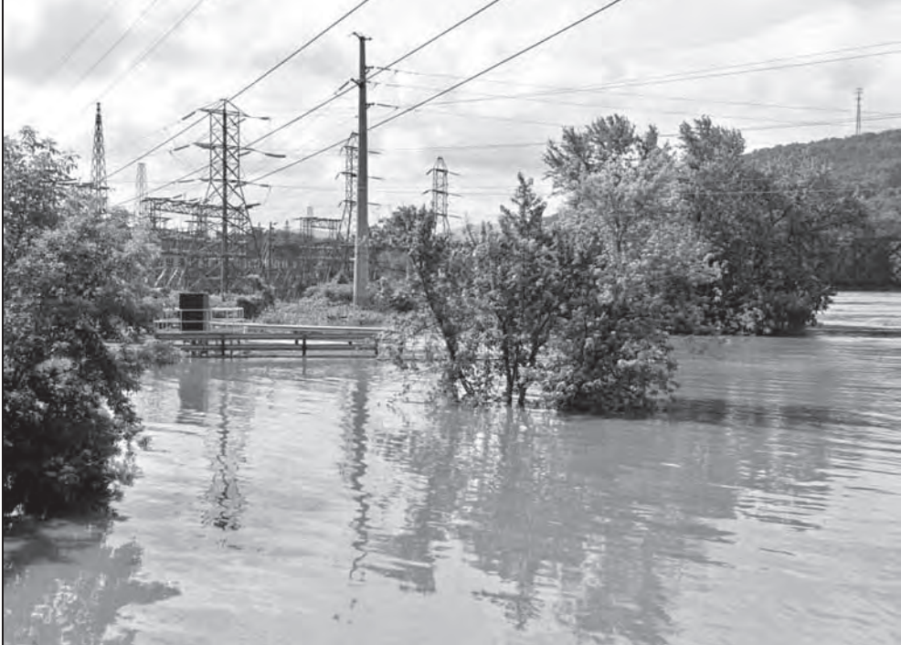
A view of control boxes for Johnson City's combined sewer overflows. In the background is the AES Power Plant in Westover, NY.
