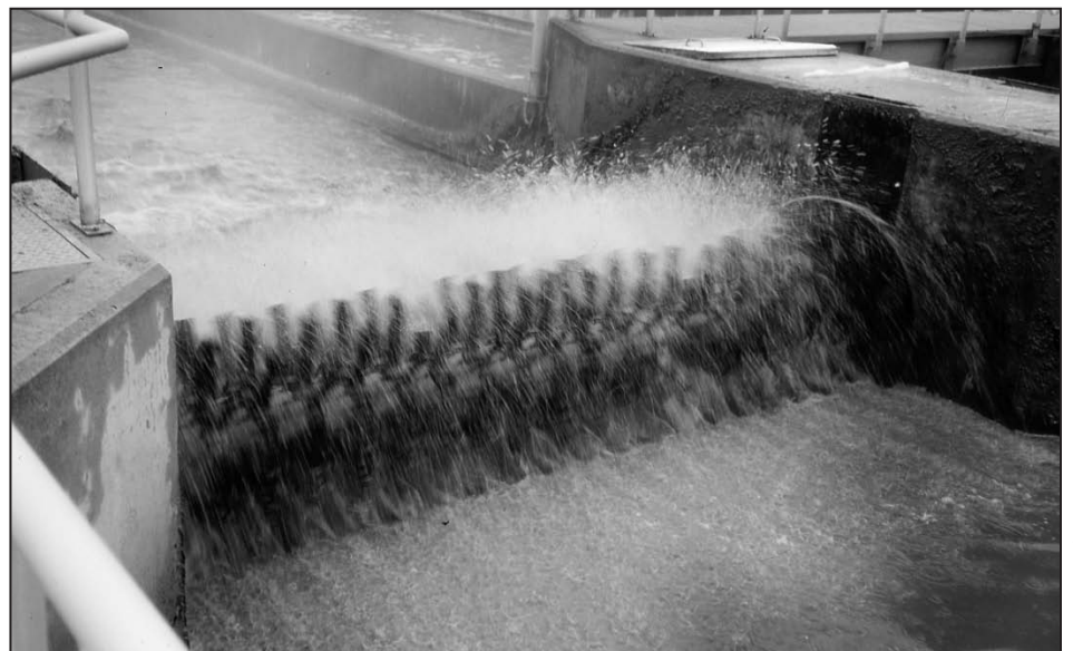
Oxidation ditch paddles must be replaced, a necessary maintenance cost.
