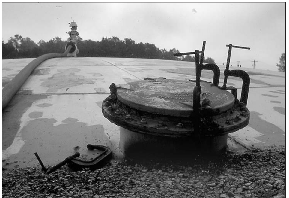
Mechanical equipment's useful life typically does not exceed 30 years as seen by this digester cover that is in need of replacement after 25 years of service.
