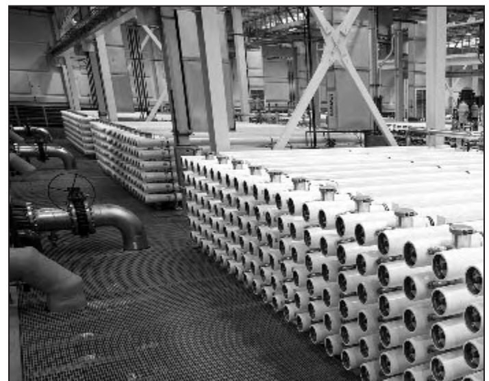
During the reverse osmosis step, applied pressure allows water to pass through tiny membranes filtering out pesticides, pharmaceuticals, and any remaining bacteria. With unwanted contaminants left behind, the resulting water is 100 percent virus free.
