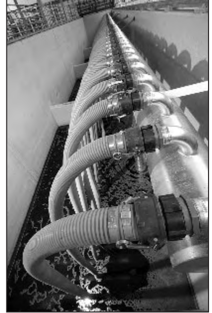
The stainless steel air manifold connects to each MF membrane module with a flexible hose. During the MF backwash operation, air is forced through holes in the bottom of the membrane modules, gently agitating or scouring the surface of the membranes to remove debris.
